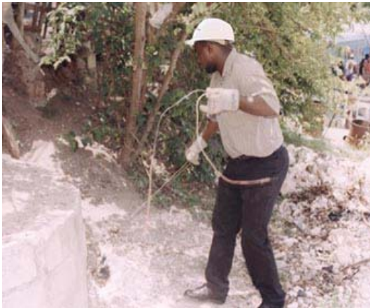
Figure 2.0 - Removal of illegal power lines (below surface) by a JPSCo member.
